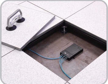
Mounting Applications – Mounts easily in tight spaces (e.g., under raised floors) for distributing fiber in a variety of applications and environments.
