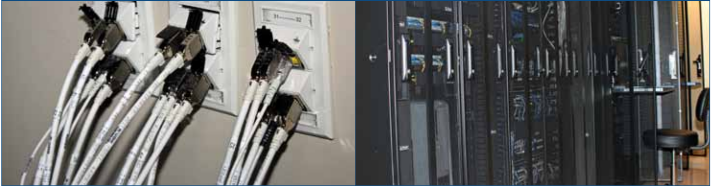
City of Rock Hill Utilities Department in South Carolina deployed cable sharing to support everything from video, VoIP and analog telephony, to CATV, video surveillance, IP radio and data.
